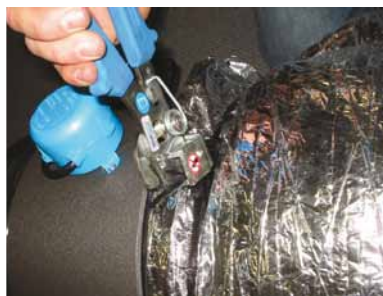
Air Condition Duct
